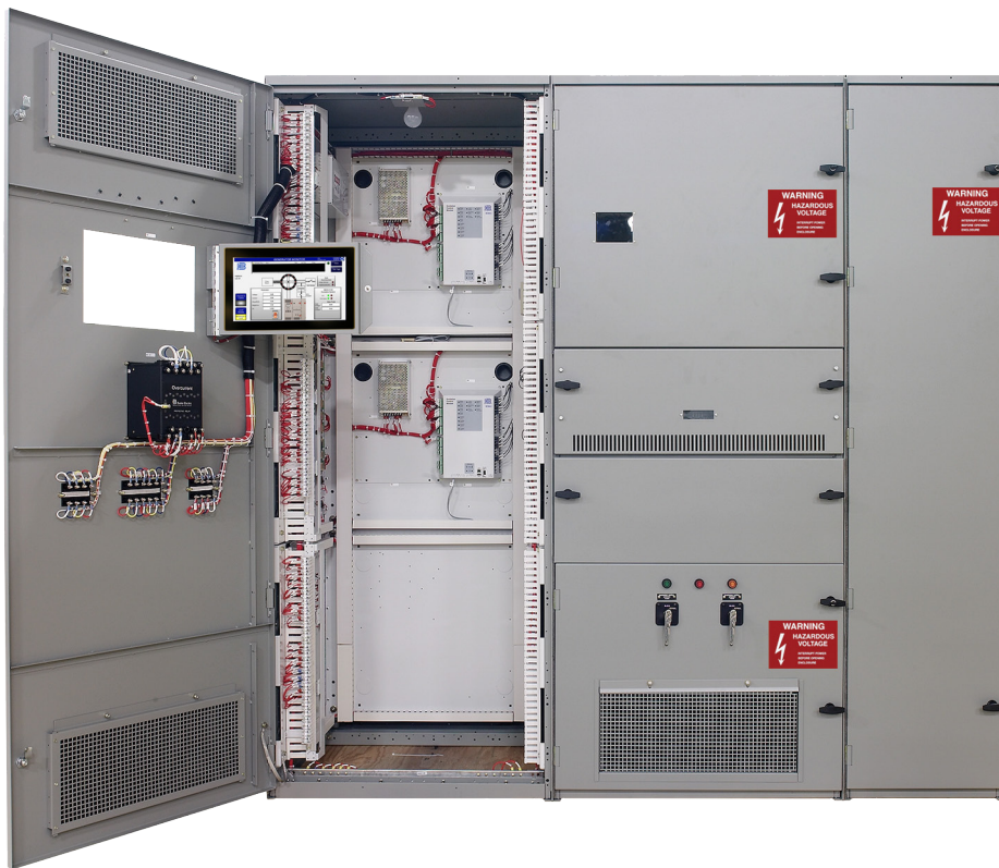
Figure 4: ECM-2 IDP-1500 installed in an excitation system cabinet
