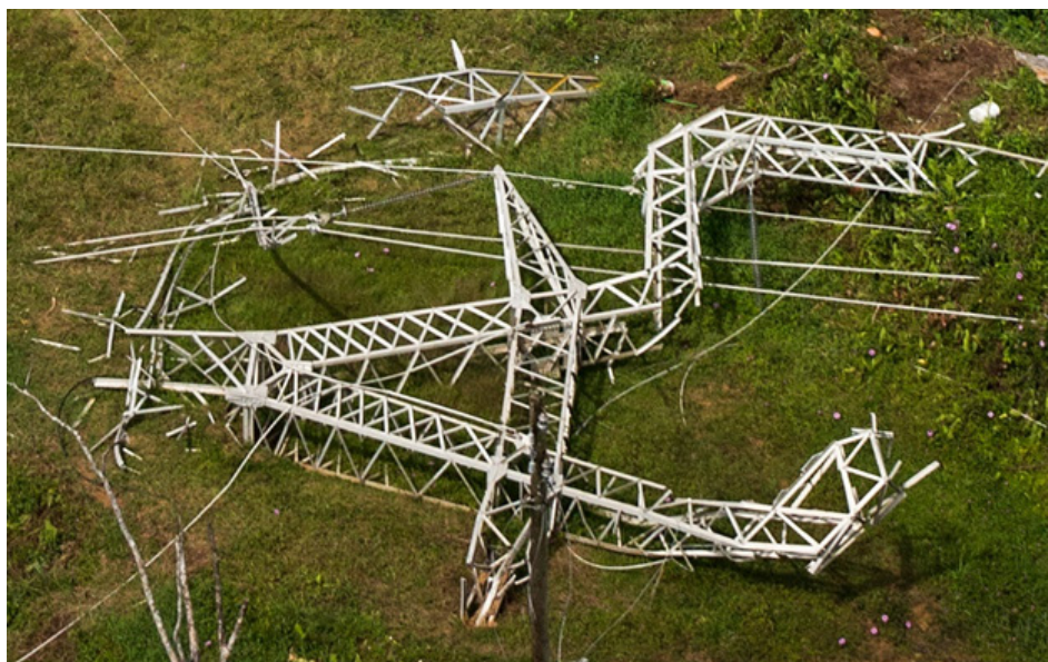
Destroyed transmission tower in Puerto Rico after Hurricane Maria [1]
