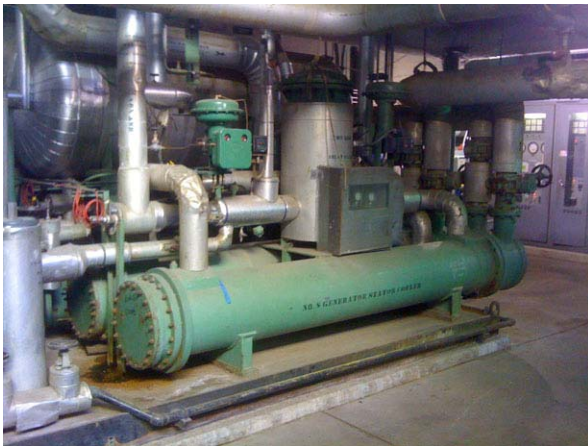
Figure 9. Generator Stator and Cooling Water System, Alterrex "In" and "Out" water lines are capped for retrofit to new Convection Cooled 2000 Amp Bridge System.
