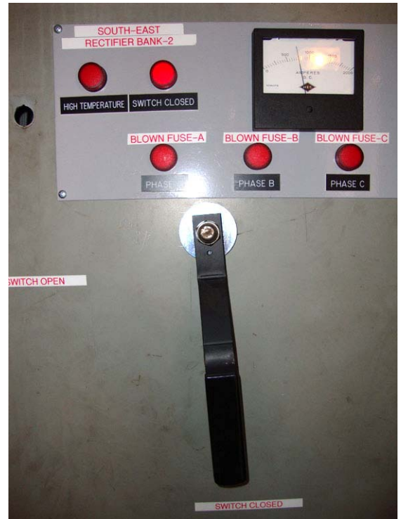
Figure 15. Display Alarm Panel and Hand Disconnect Switch
