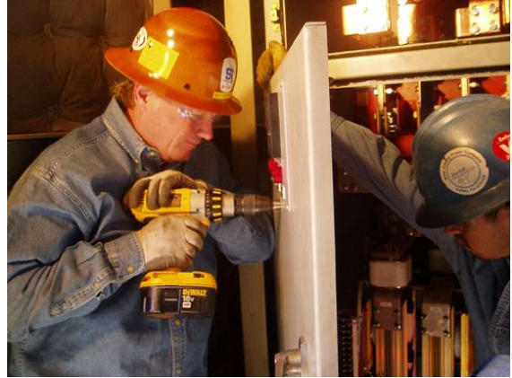
Figure 14. Center Hole for Outside Disconnect Switch drilled by local electrical contractor Technician Sermco Industries
