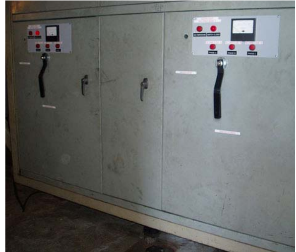
Figure 16. System Line-up of the SW Panels with Rectifier Panel Doors Closed
