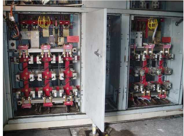
Figure 1. Old Water-Cooled Bridges
