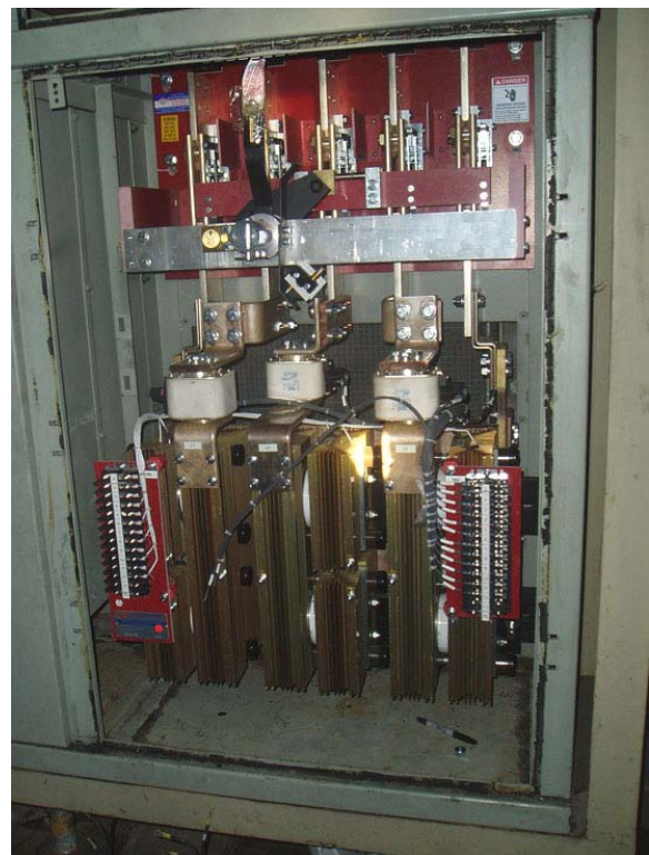
Figure 11. New Bolt Action Disconnect Switch and Convection Cooled Bridge
