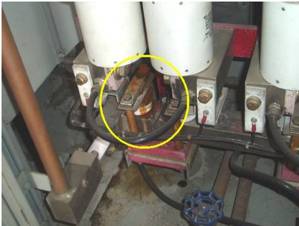
Figure 2. Corrosion tracking of leaking water
