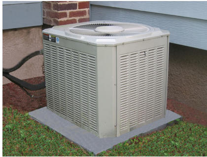
Commercial and Residential HVAC Equipment
