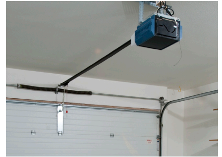
Garage Door Controls
